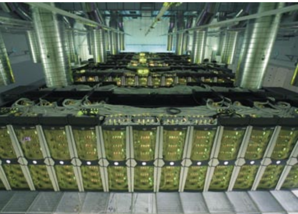
Figure 1: SGI 4700 during installation
